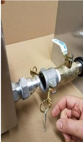
Pump to Valve
